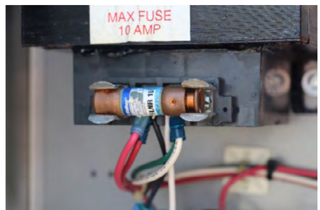
Figure 3. The fuse inside the main control panel.
